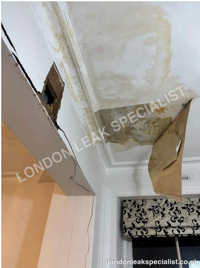
Photo 1. Ceiling opened where water was coming through in the flat below, with the boxed-in steel beam beside it.
