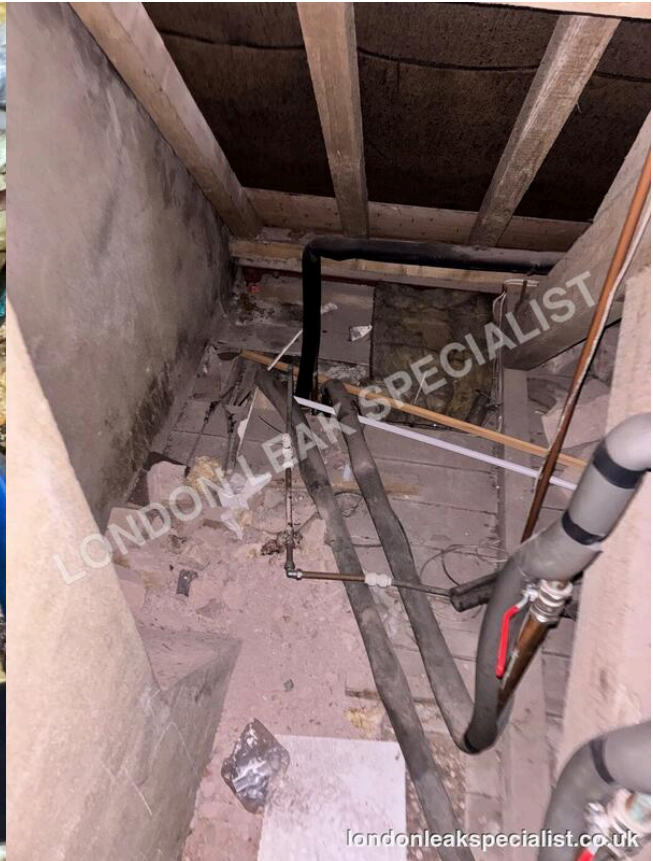
Photo 6. Lagged pipework and valves in an accessible void.
