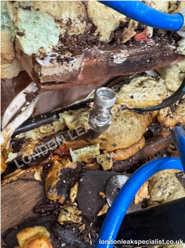
Photo 5. Damp debris and an isolation valve where bathroom fittings had been removed.
