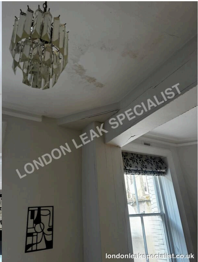
Photo 2. Water staining on the ceiling of one of the affected flats.
