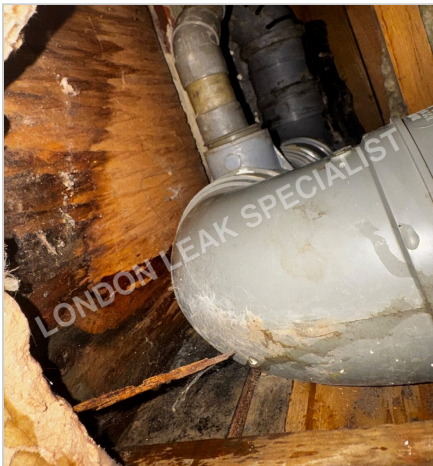
Stack, branch connection and water-stained timber in the void
