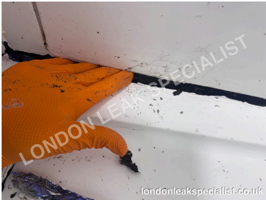
Photo 2. Failed mastic and an open joint at the shower tray edge.
