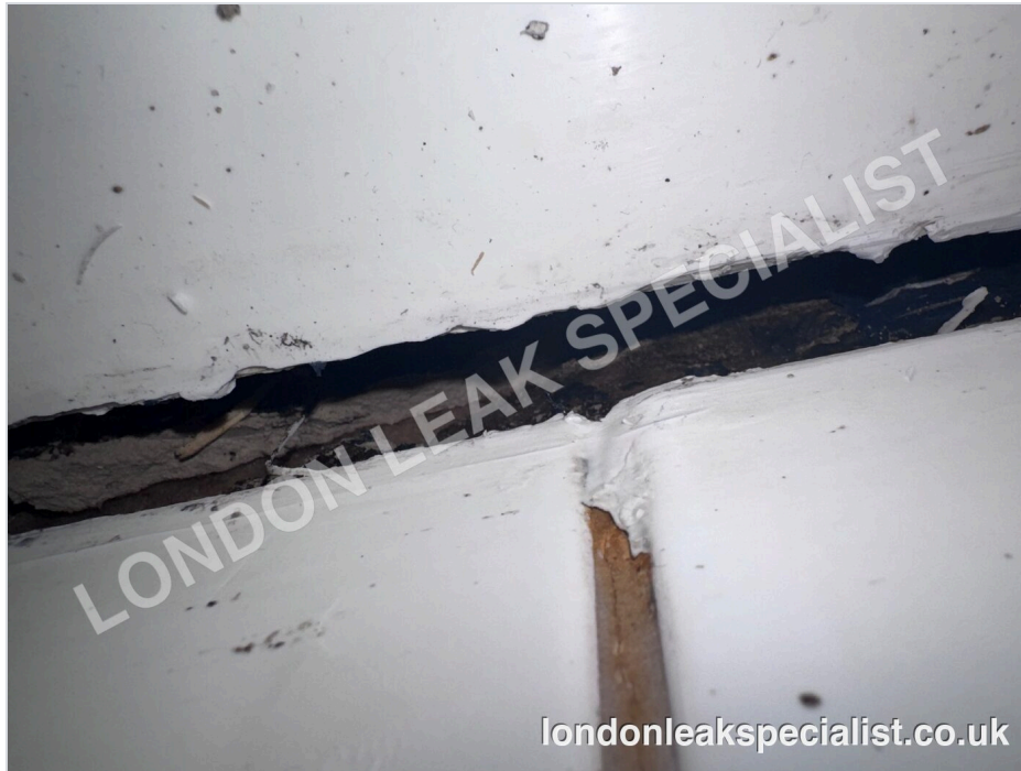
Photo 3. Opened joint at the tray, with the timber beneath visibly stained.
