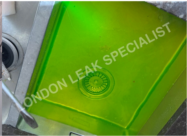
Photo 2: Tracer dye run through the kitchen sink
