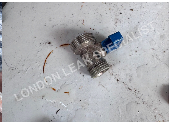
Photo 6: The defective valve after removal
