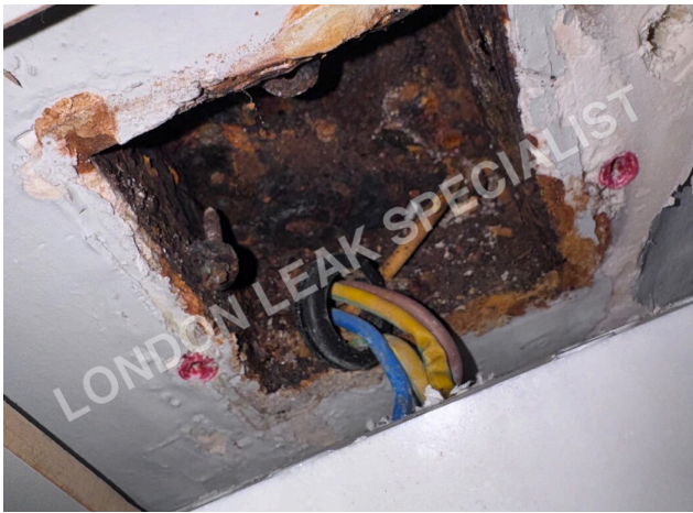
Photo 1: Corroded back box of the wet socket that first raised the alarm
