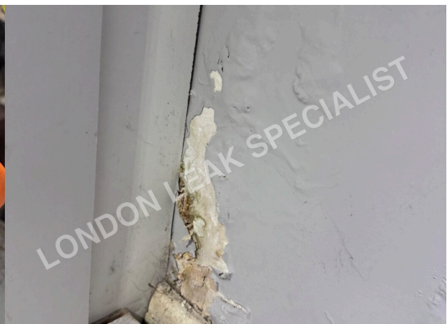
Photo 4: Salt and paint damage along the rear kitchen skirting
